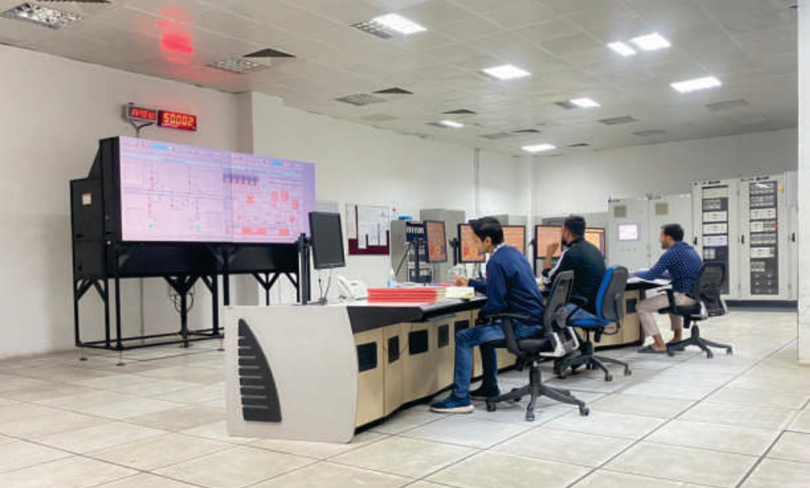
Control Room - Sainj HEP 100 MW
