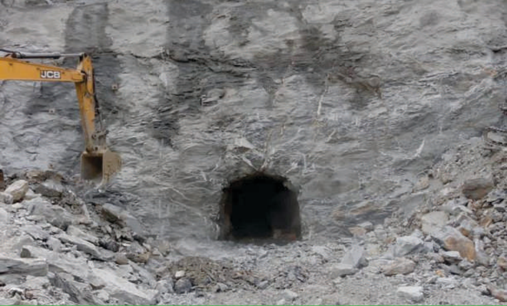
MAT Portal Showing Drift - Chanju III HEP
