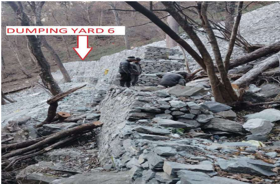
Fig. No. 5 – Dumping Site 6
