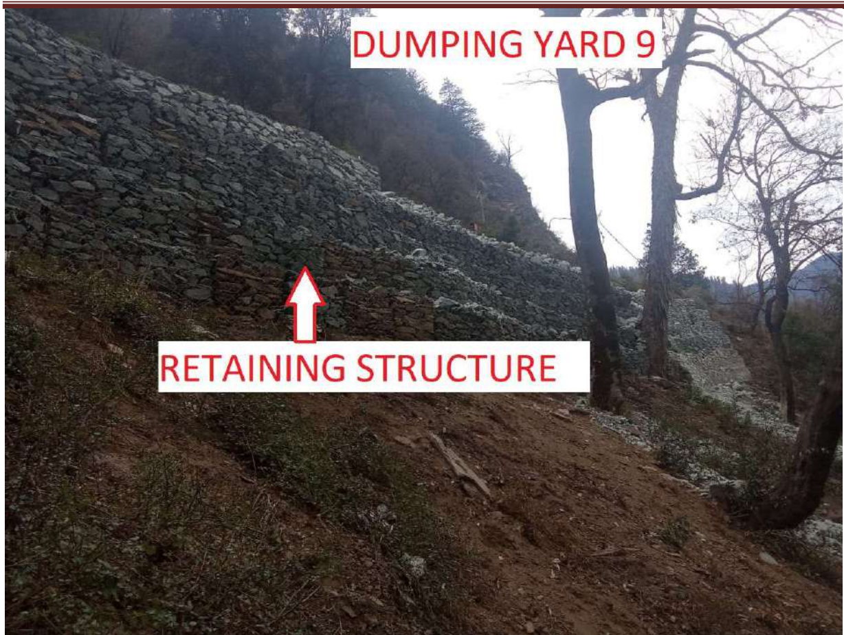
Fig. No. 7 – Dumping Site 9
