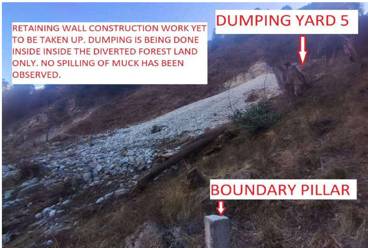
Fig. No. 4 – Dumping Site 5
