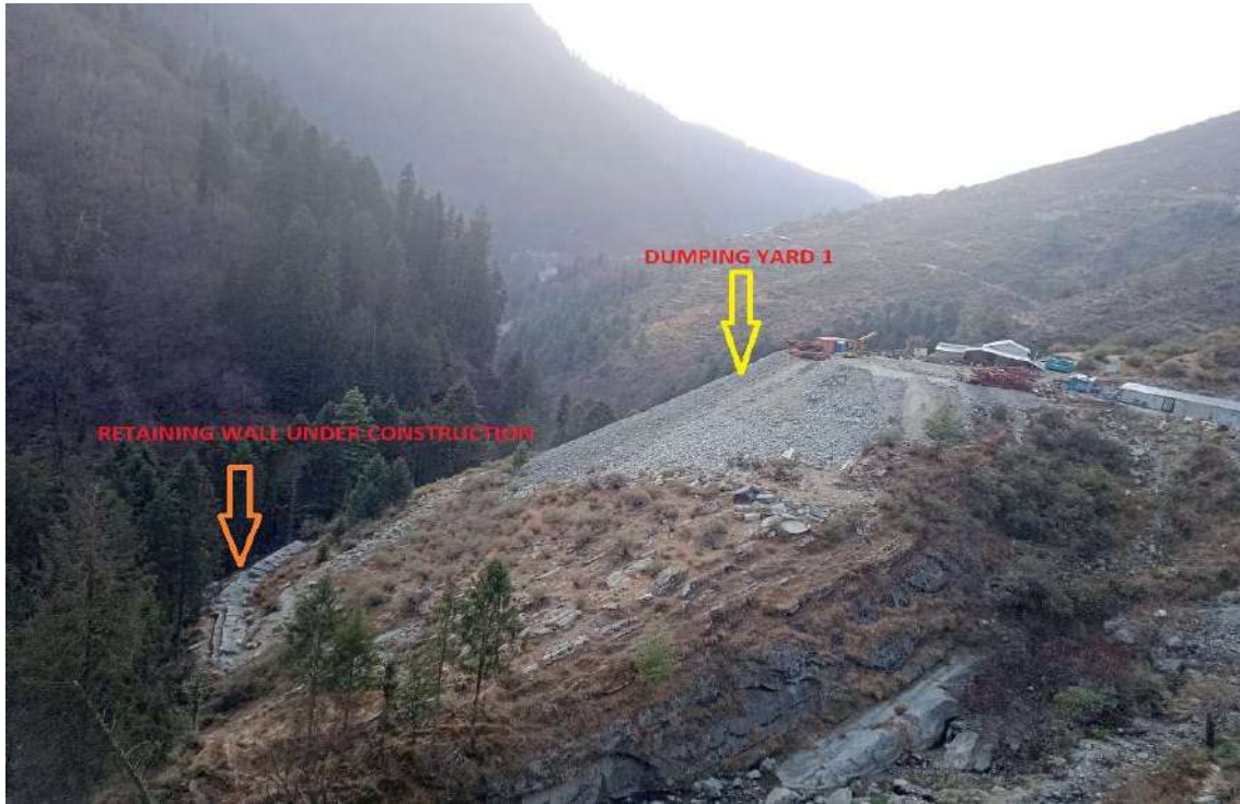
Fig No. 1 – Dumping Site 1
