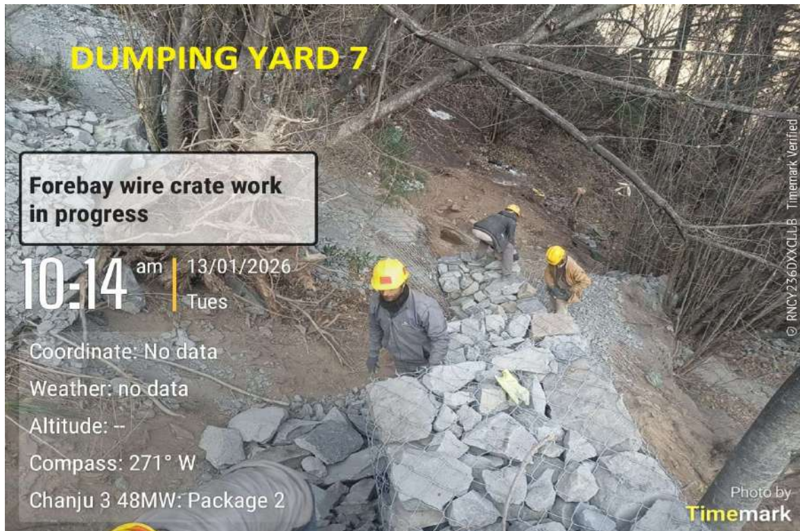
Fig. No. 6 – Dumping Site 7
